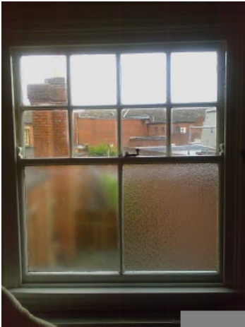
All Windows in Room, Window frame/sill, Window glass, Curtain Hooks, Curtain Rail
