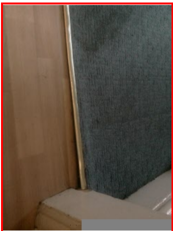
Floor - Carpet not fastened down with door strip properly (moderately)
