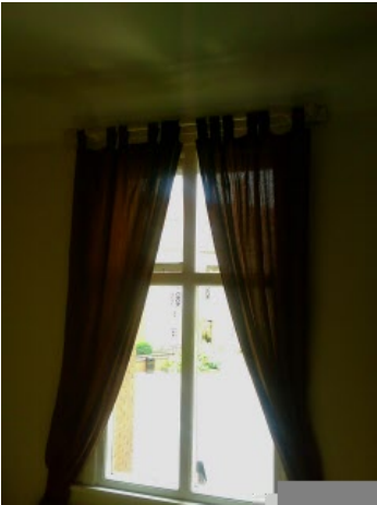
All Windows in Room, Window frame/sill, Window glass, Curtain Rail, Finials, Unlined curtains
