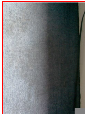
Floor - stained (in several places)
