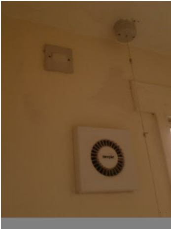
Extractor Fan, Light Switch, Wall Finish, Fused Switch
