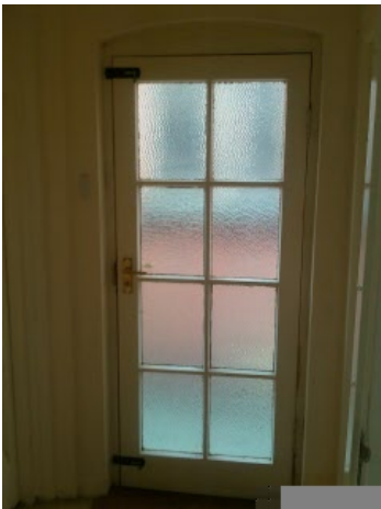
All Doors in Room, Door Finish, Door Frame, Door Glass, Handle, Lock
