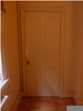
All Doors in Room, Door Finish, Door Frame, Door Glass, Knob, Hinge
