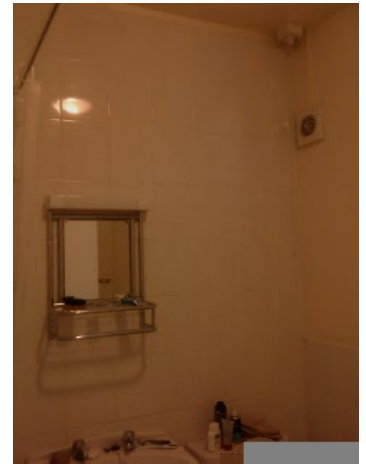
Wall Finish, Bathroom Mirror, Extractor Fan, Fused Switch, Shelf
