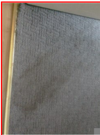
Floor - stained (in several places)
