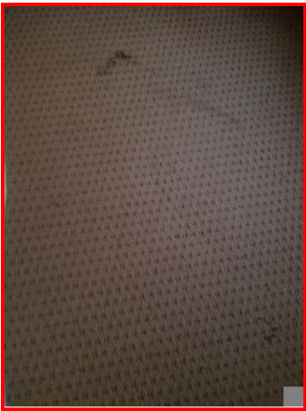
Floor - stained (in several places)
