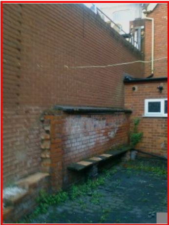
Boundary/Partition - damaged (Damage to wall due to age)
